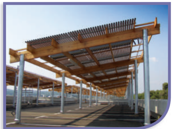
Solar Cooling in Galderma Pharmaceutical Research Centre, France. The 5,600 tubes double up as a car park pergola.
