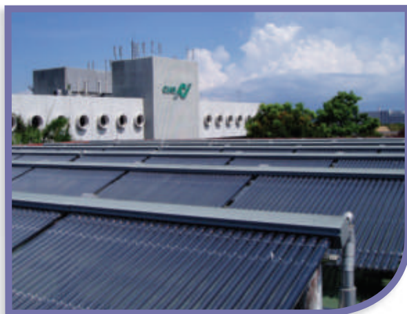
Changi Airport, Singapore. Largest solar thermal installation with more than 10,000 tubes.
